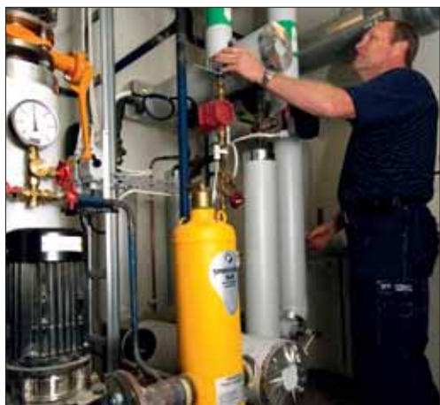
District heating, Maskinkajen
